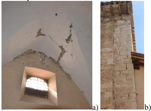
Fig. 9. a) Cracks in the cross vaults, b) detachment of the façade from the lateral bearing wall
