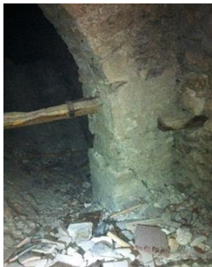
Fig. 10. Serious crack at the abutment of the arch in the area near the old wooden tie.
