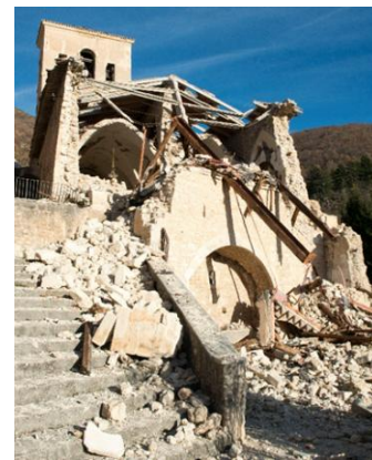
Fig. 12. St. Andrew's church: state following the 30 October earthquake
