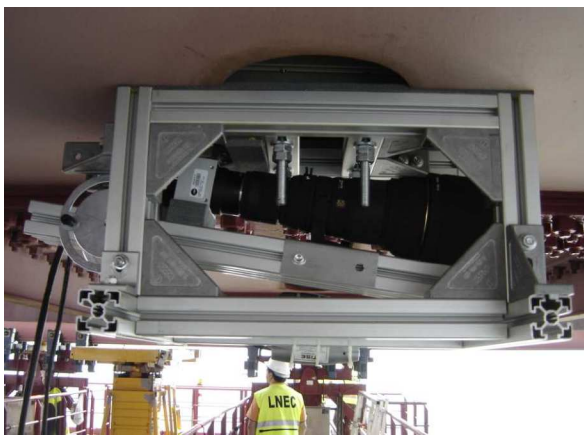
Fig. 3. Digital camera installed in the stiffness girder
