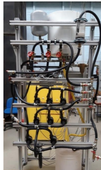
Figure 5-6. Application endurance test stand for 12 DUTs
