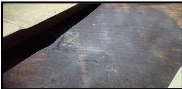
Fig-4: Broken and burn marks were found on permawood ring of coil support platform.
